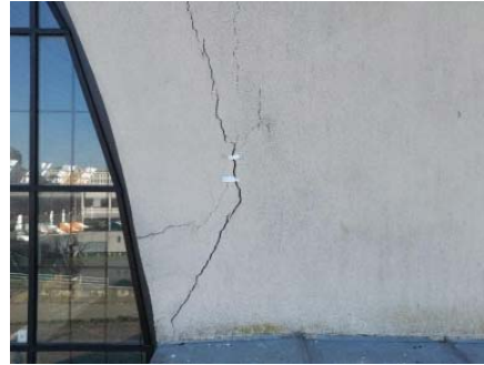
Fig. 2. Cracks in the North Face of the Dairy Pavilion (Māris Strazdiņš 2024)
