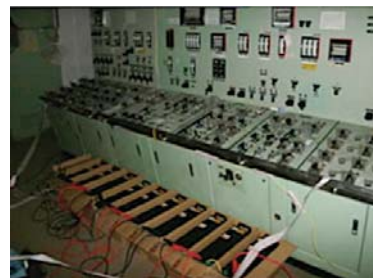
Fig. 1. A famous instance of adaptive decision-making: due to total loss of power, the Fukushima Daiichi nuclear power plant operators used car batteries as power source for the instruments. Foto: Tepco. https://www.tepco.co.jp/en/nu/fukushima-np/review/review1_2-e.html
