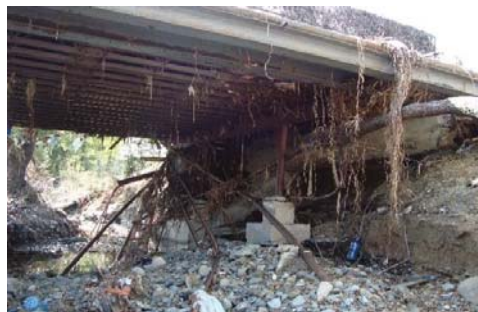
Fig. 4. Bridge – “Mandrata” – damages
