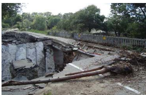
Fig. 3. Bridge – “White shore” – damages
