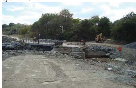
Fig. 5. Bridge – “Coastal Alley” – damages
